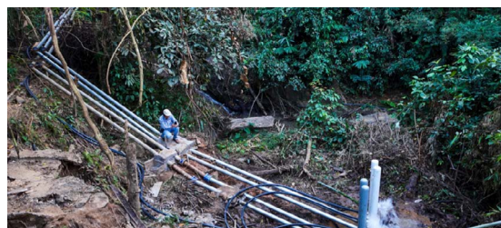
Water inlet and hydraulic pump
